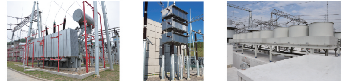
Coupling transformer Charging resistor Water cooling system
